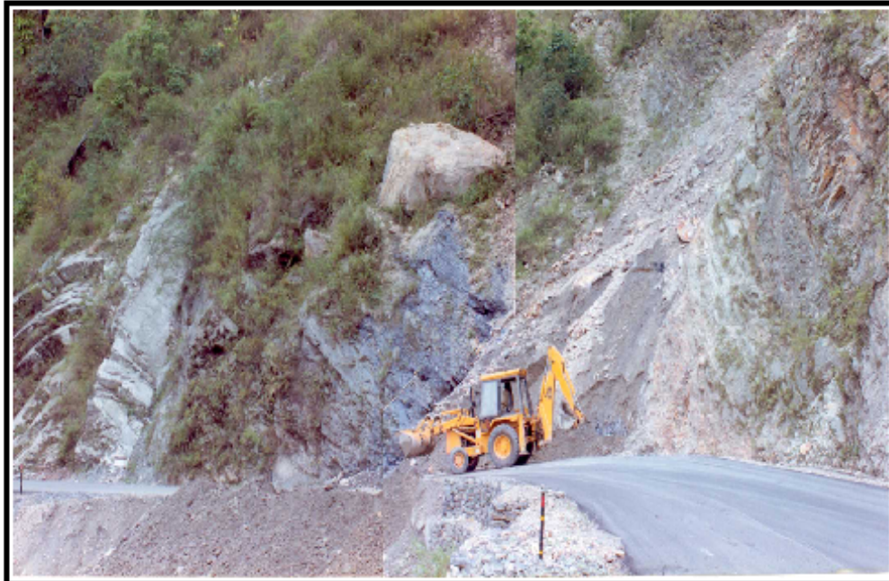
Plate 2.16 Berrick landslide showing a fault propagated fold and the circular failure of carbonaceous phyllite
