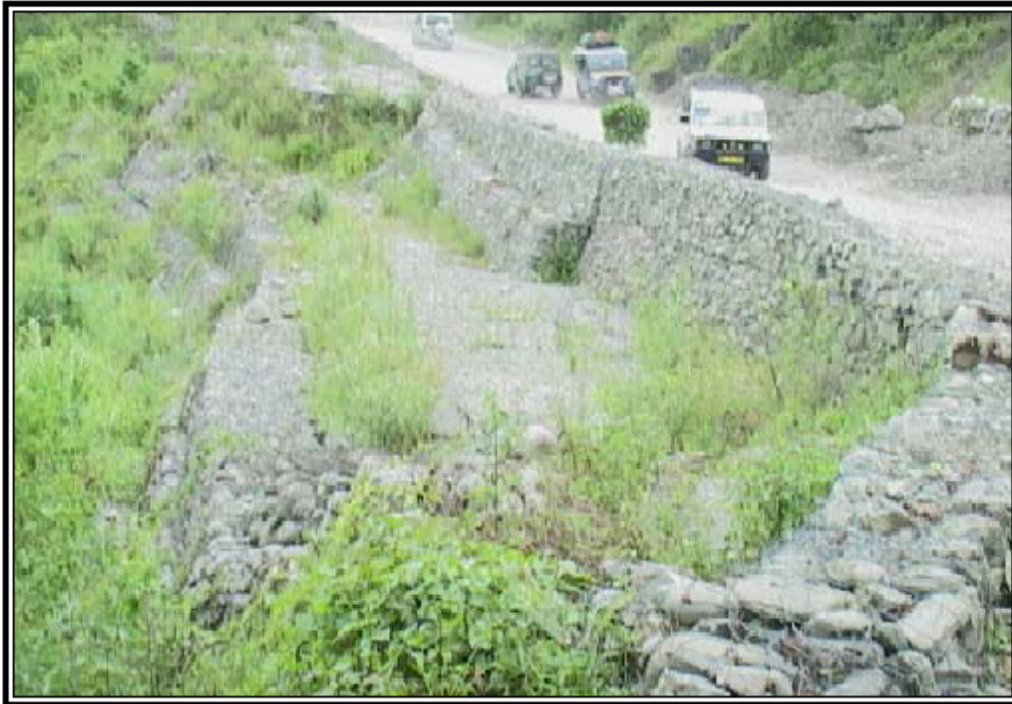
Plate 2.11 Creeping and collapse of the protection wall near Ri Chhu
